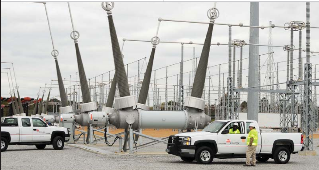
Entergy Mississippi will invest $45 million in a project at the Ray Braswell substation in Clinton, Miss. that will improve reliability for customers from Jackson to Brookhaven. Gene Hodges and Ronald McMorris (in truck), both operations coordinators with Entergy Mississippi, Inc., discuss a work project while in front of the transformer at the substation.
