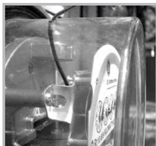
Customers who divert electricity run the risks of fire, shock, and even death.
