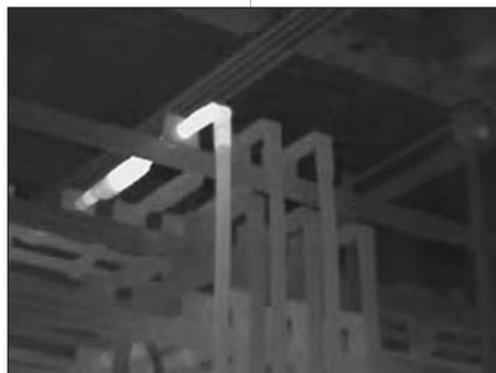
The image above shows an example of an infrared equipment reading that demands immediate attention. The brightest part of the image indicates the highest temperature.
