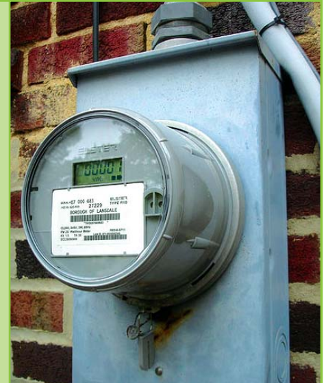
The photo above shows an example of a newer retrofit US domestic digital single-phase smart meter.*
